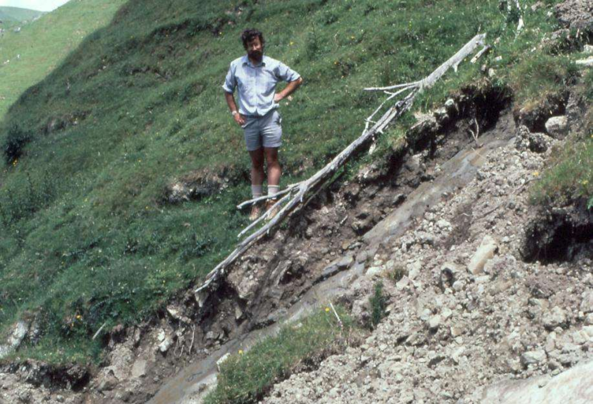
Note the sharp boundary between the soil and underlying rock, forming a slip plane.
