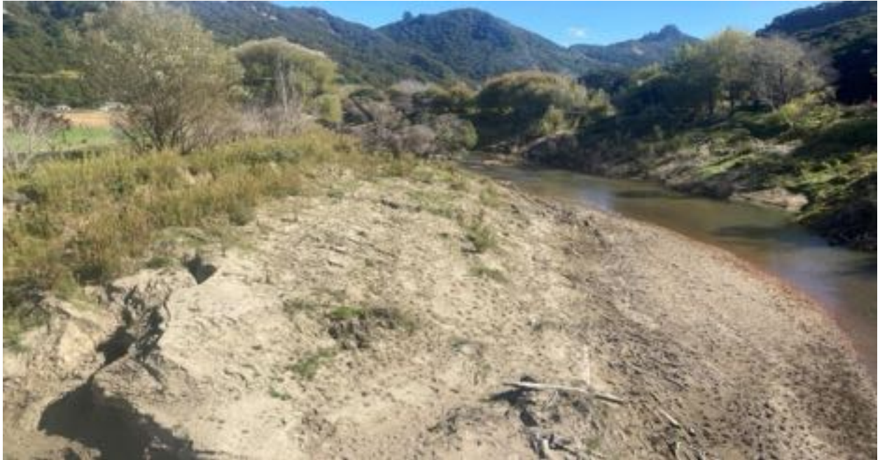
Figure 25. View of Hikuwai River showing stable sloping banks. Overland flow returning to the channel caused the erosion in the foreground.
