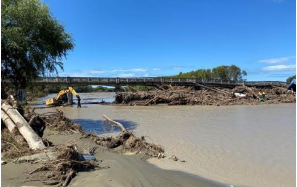
Figure A36. Woody debris on collapsed Redclyffe Bridge.
