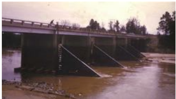
Figure A38. Bridge debris fins.
