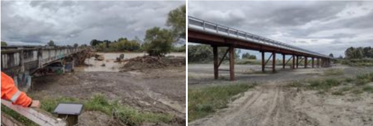
Figure A22. Redclyffe Bridge – cyclone debris removal (left). Redclyffe Bridge – interim repairs (right).
