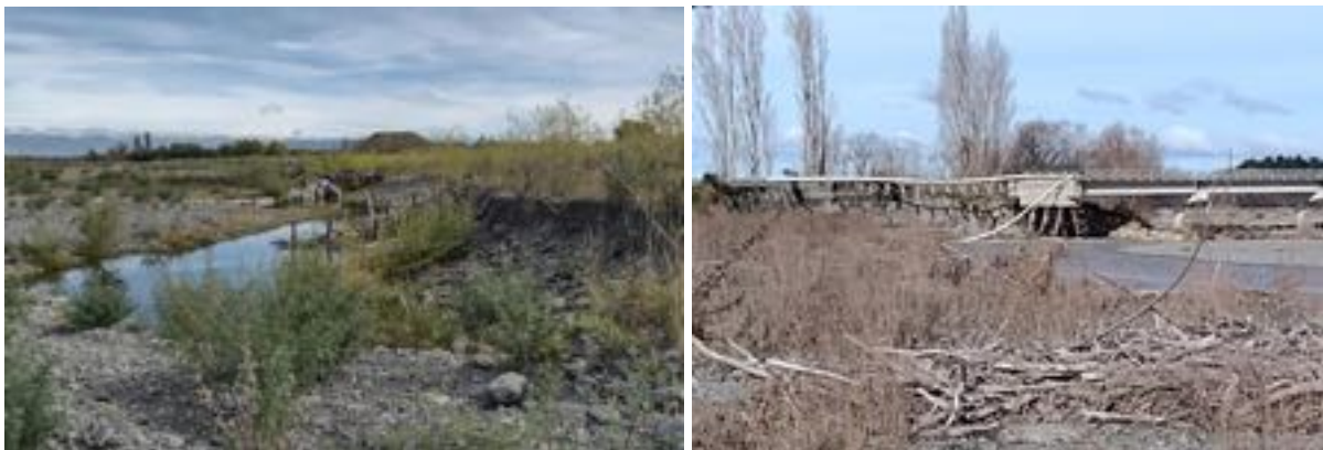
Figure 16. Bank erosion with damaged Akmon & rope/rail groynes (left). SH50 Bridge wash out (right).
