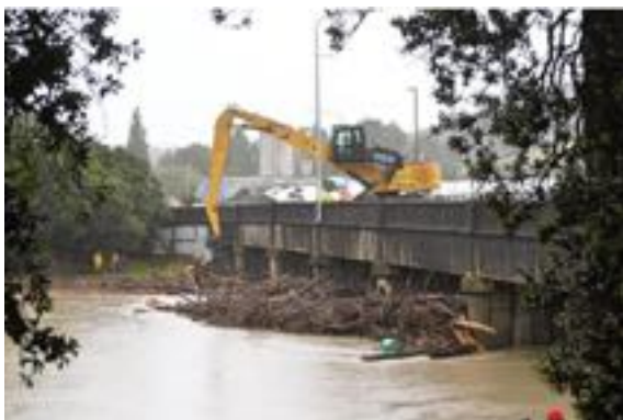
Figure A37. Woody debris removal during flood.
