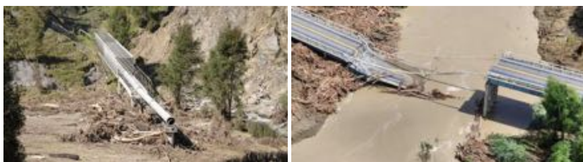
Figure A23. Damaged Gisborne water supply pipeline & Hikuwai No.1 Bridge.
