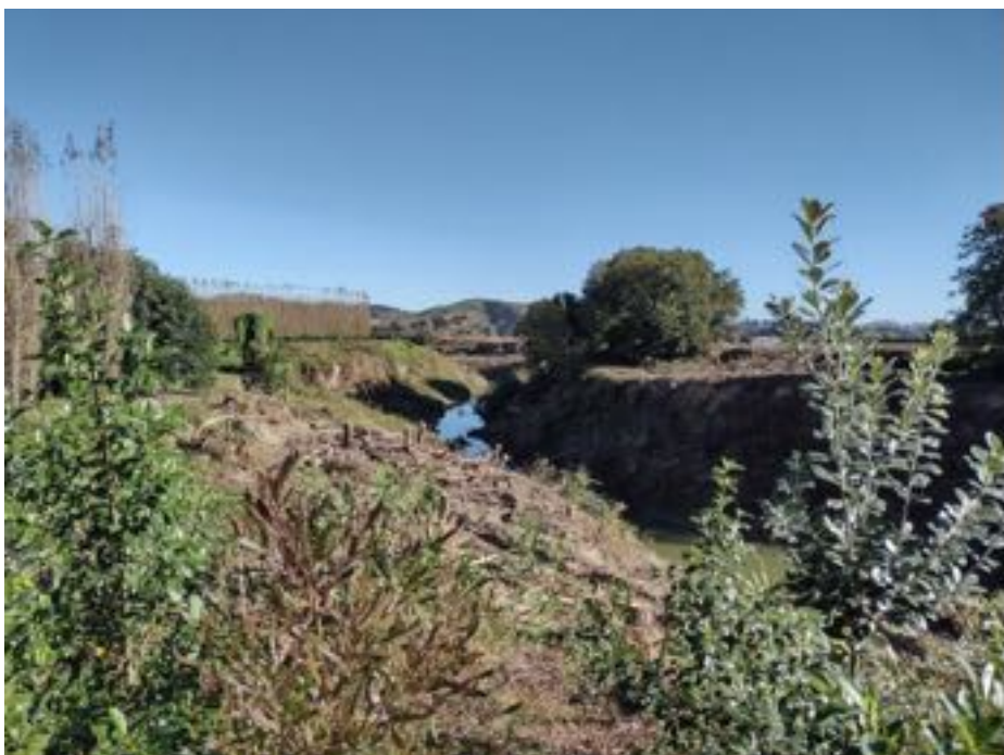
Figure A31. Te Ārai River – results of extensive channel debris clearance & tree removal works post Cyclone.
